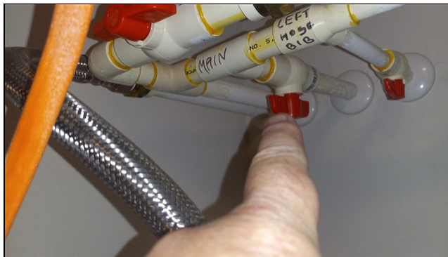
main water shutoff
